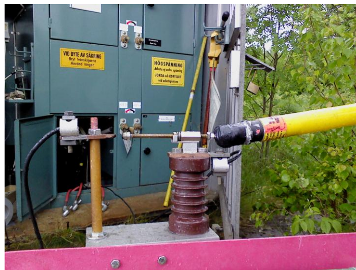
Picture 3: Intermittent fault by “decreasing air gap” method
