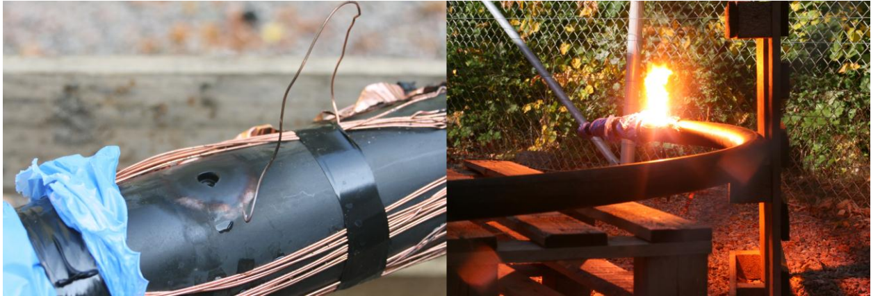
Picture 2a & 2b: Intermittent fault by “drilling hole and pouring water” method
